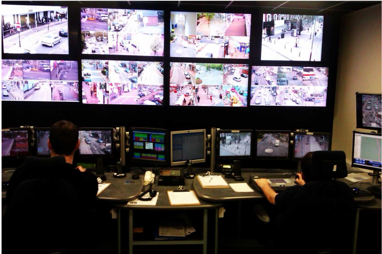
CCTV Control Room
